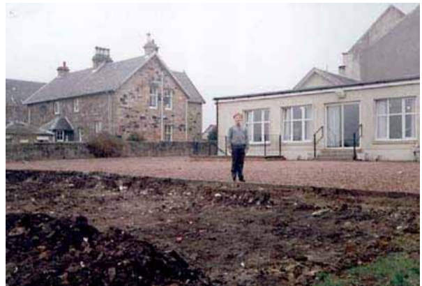
Heavy machinery was needed to clear the site Mr Clark, Mr Walker and Mr Gibson helped in various ways to excavate the land.
